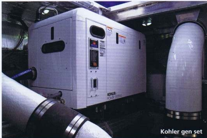
The engine room, while tight, still affords room for servicing
